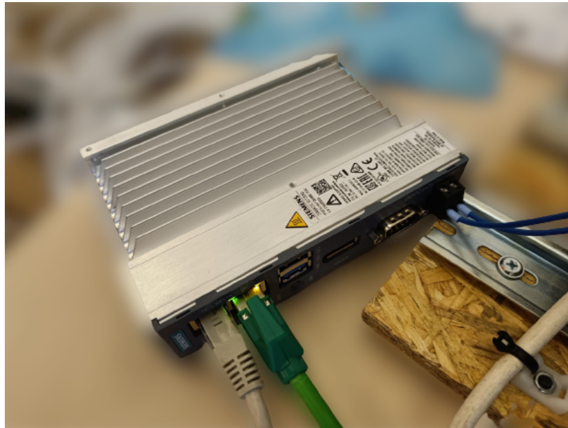
Figur 4. Siemens Simatic IOT2050 i drift.
